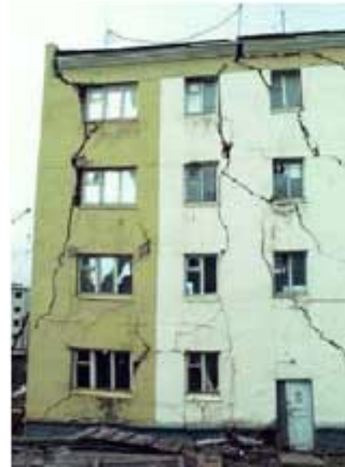
Figure 1. A building that has buckled due to thawing permafrost. — Credit: Vladimir Romanovsky, UAF
