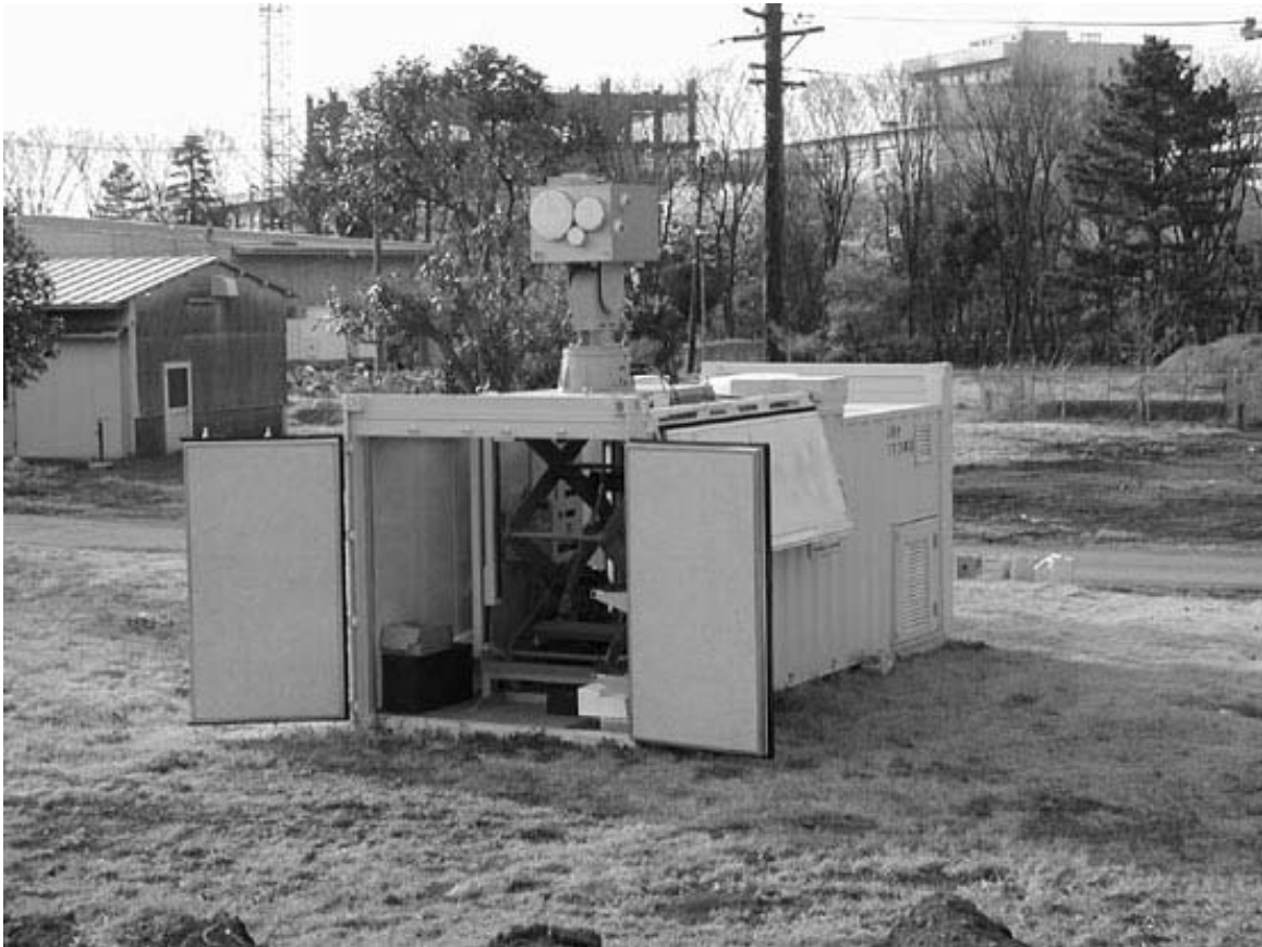
Figure 21. Ground Based Microwave Radiometer (GBMR-6Ch) system.
